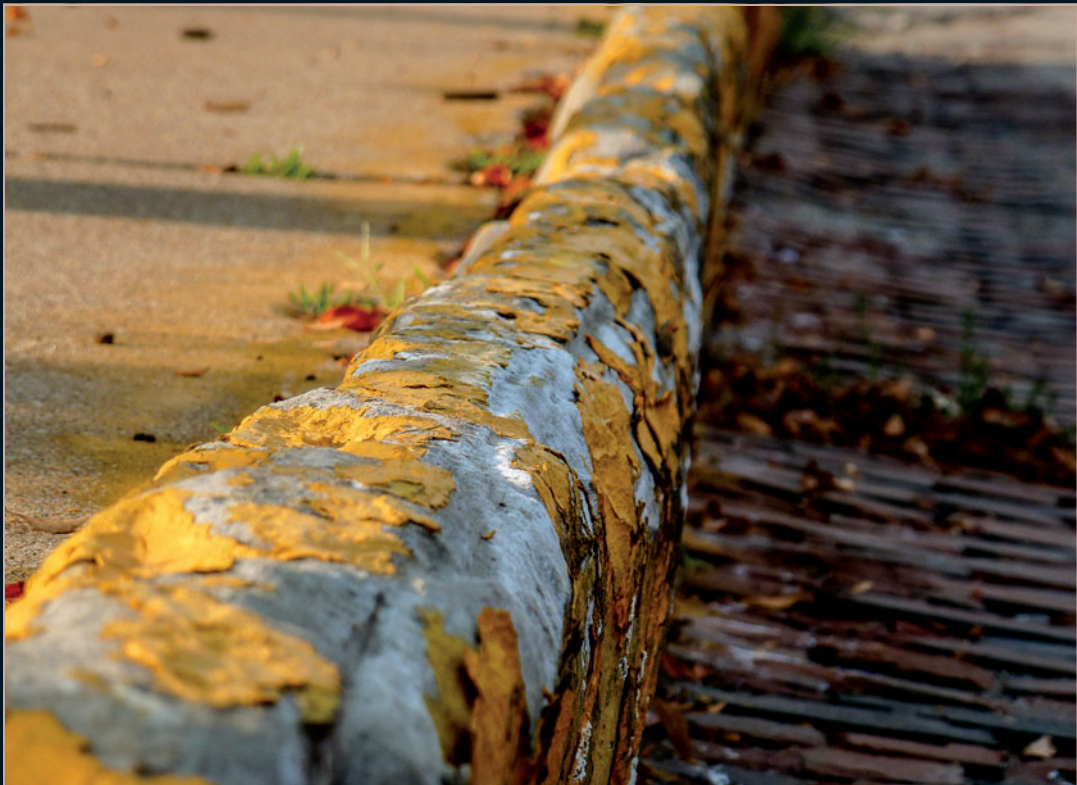
Paint peeling from a curb
