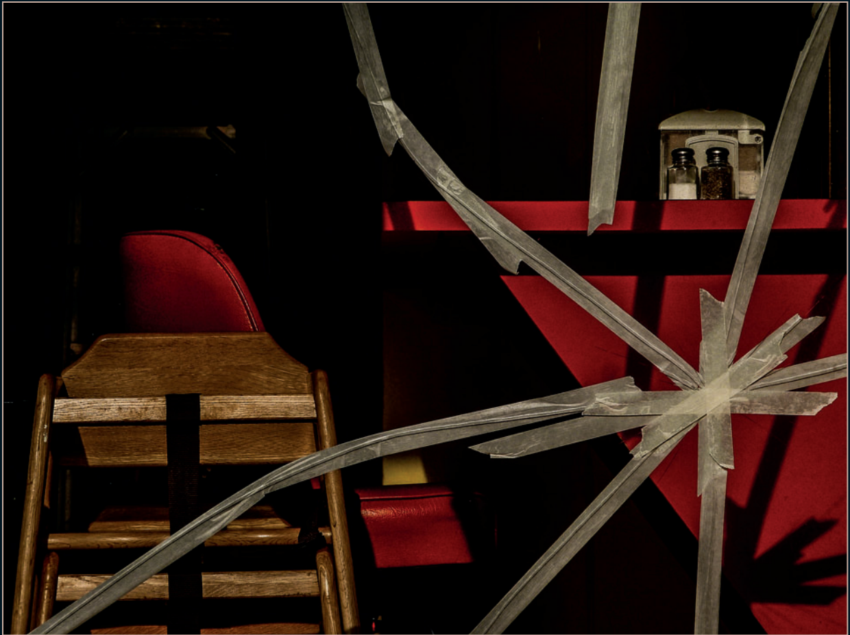
Broken window. The tape made for an interesting layer over the initial composition.
